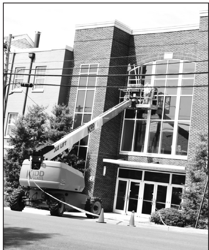
WINDOWS WERE REPLACED at Versailles Baptist Church last week. On Wednesday afternoon, April 8, workers used a lift to reach the windows being replaced on the part of the church building that faces East Green Street in downtown Versailles. In September 2023, Versailles Baptist's steeple was lowered to East Green Street for repairs. (Photo by Bob Vlach)
