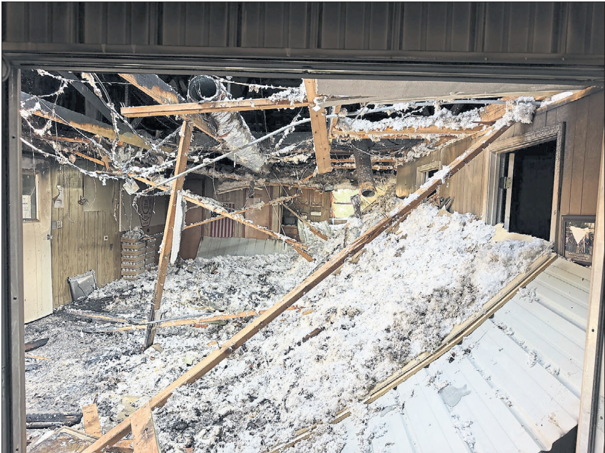
The interior of the Cuba Volunteer Fire Department sustained significant damage.
