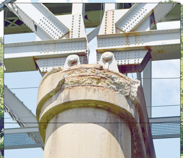
▲ PHOTO | MARY BETH SALLEE Concrete spalling is visible at the top of a pier beneath the US 31W bridge over Green River. While the condition is not a structural concern, it is cautioned against standing directly beneath the pier because additional concrete could flake off.
