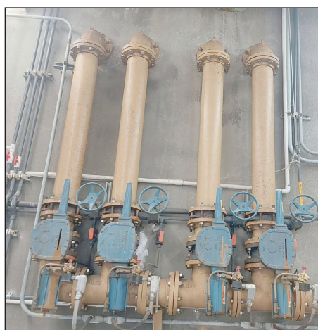
▲ PHOTO | LYNN BLEDSOE Part of the new water monitoring system.
