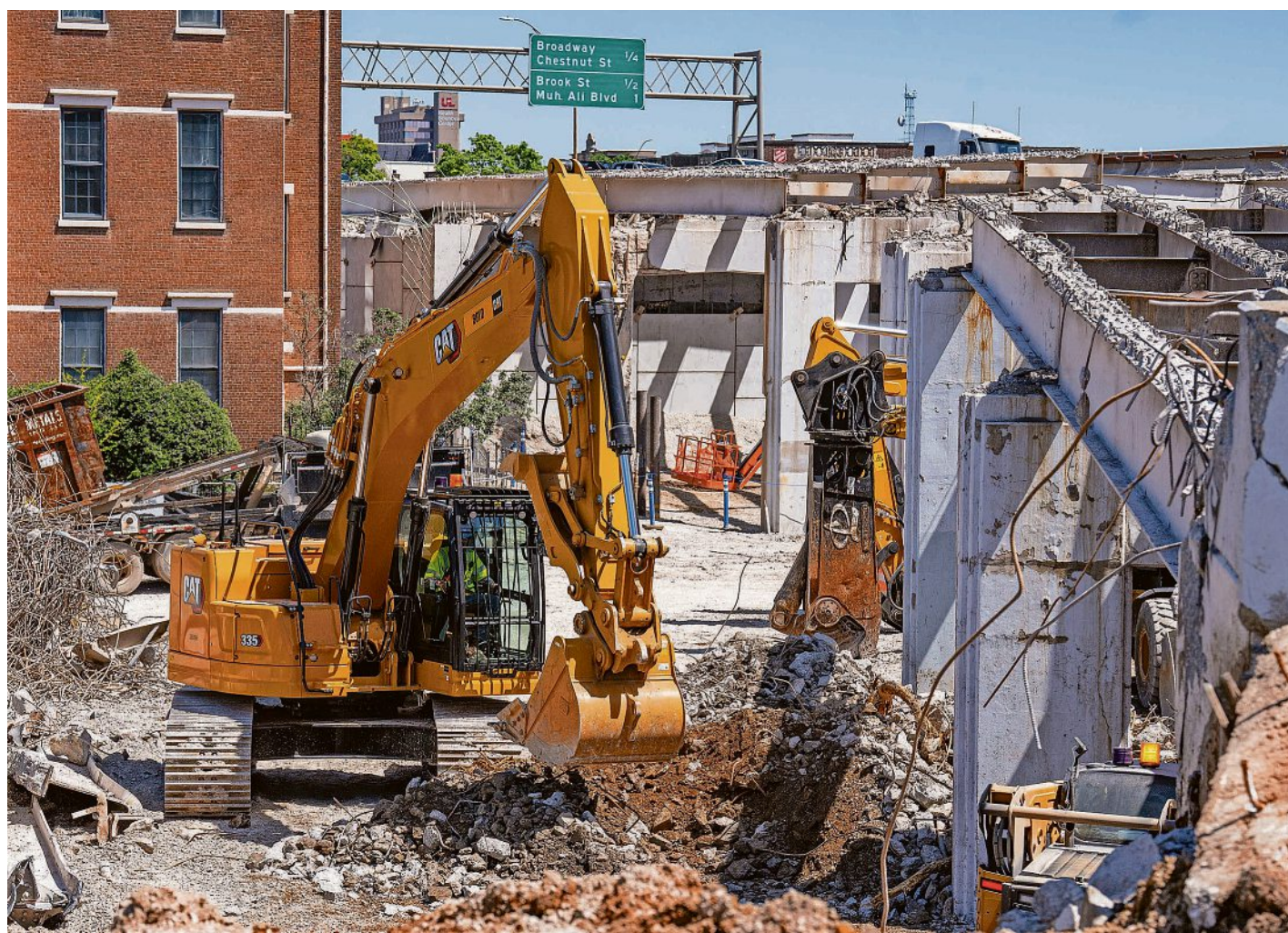
Construction crews work on the off-ramp from southbound Interstate 65 to East St. Catherine Street in Louisville on May 7, as part of the I-65 Central Corridor project ahead of a planned interstate shutdown this summer.
