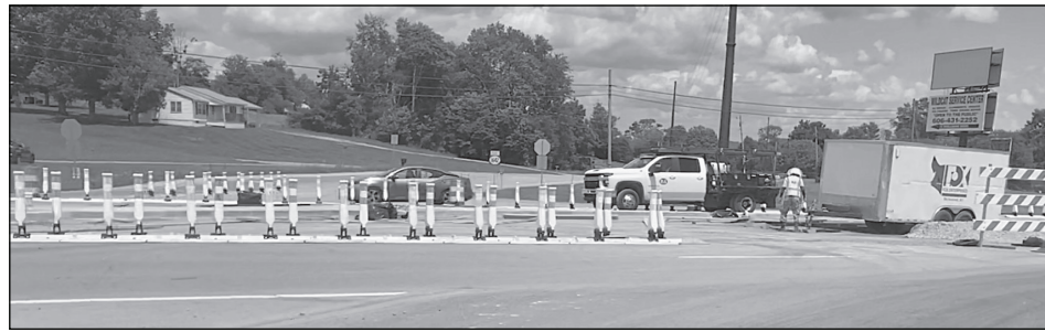
COURTESY OF KYTC Work along the Ky. 914/Slate Branch intersection is scheduled to be completed by July 31.
