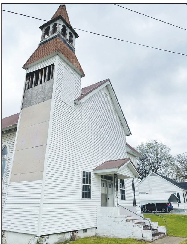
The church structure was damaged during a rough wind storm in 2023.
