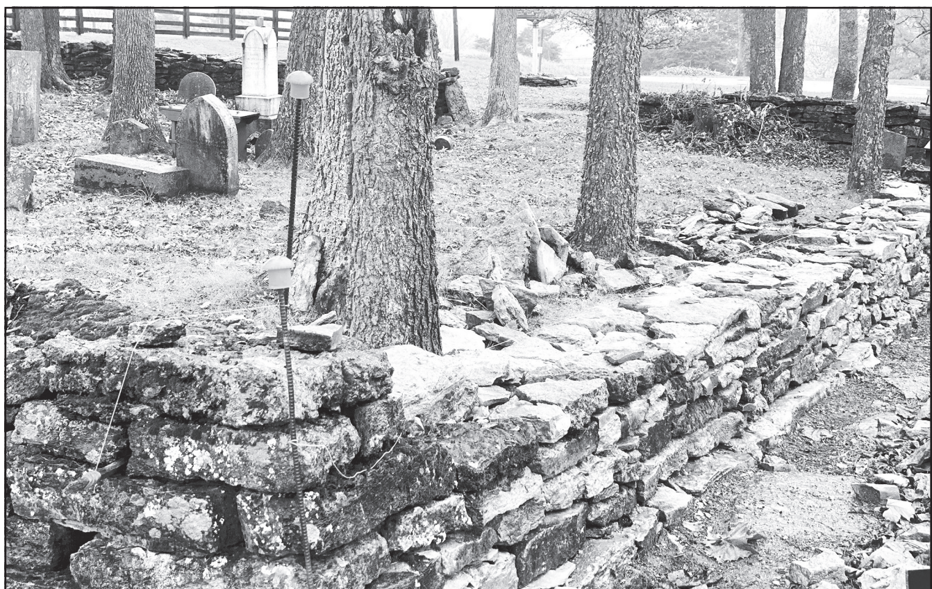
THE JACK JOUETT HOUSE’S historic dry stone cemetery wall is being restored and preserved via a joint project of the Woodford County Extension Master Gardeners, dry stone mason Keenan Bishop and other community partners. (Photo by Scott White)
