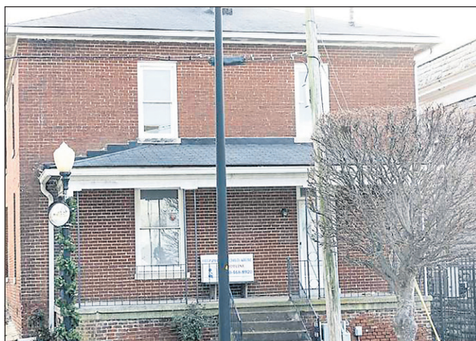
Demolition of the old jailer's house on Friday makes room for additional office space for the Washington County Clerk's office.
