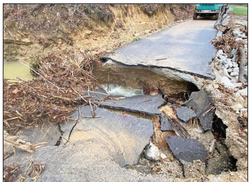
Sam Richmond/LEWIS COUNTY HERALD Heavy rain from storms moving throughout the area last week resulted in damage in portions of the county and across the state. Raccoon Branch Road was one of the roadways damaged in the event.
